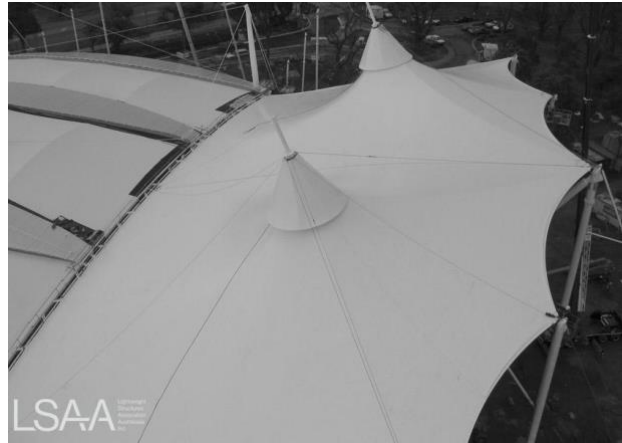
Figure 37. Roof structure of the Melbourne Sports and Aquatic Centre, Albert Park (Source: LSAA.org).
