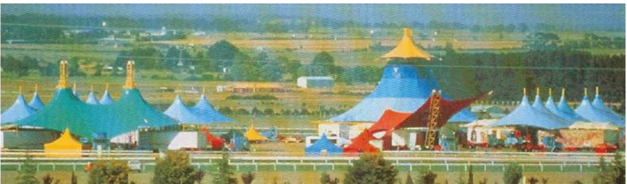
Figure 20. A full-scale trial of the erection of the Bicentennial Travelling Exhibition in Ballarat, Victoria (Source: MSAA, No. 4 1988).
