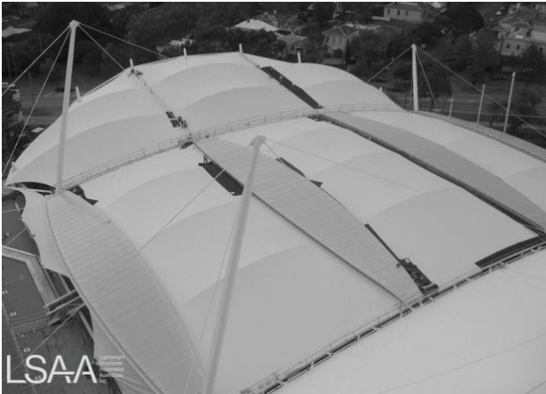
Figure 36. Roof structure of the Melbourne Sports and Aquatic Centre, Albert Park (Source: LSAA.org).
